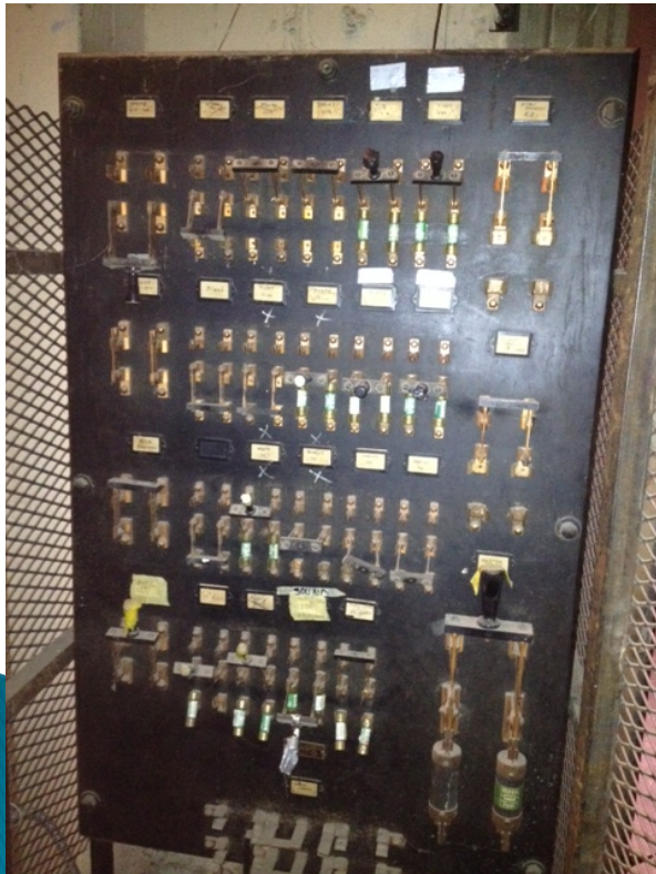
Old Knife Switch Electrical Panel
