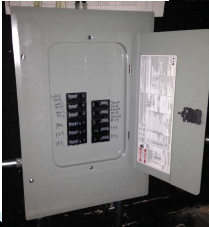
New Modern Electrical Panel
